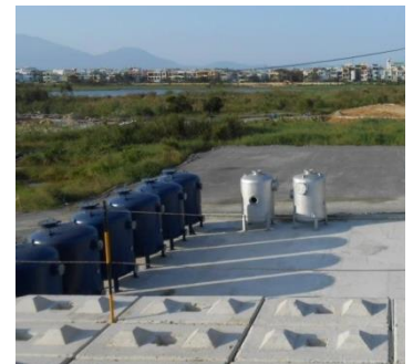
GAC vessels delivered to site (Photo: CDM Smith)
